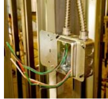
7. Electrical 7a. Permit Info
